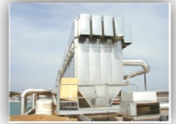
A large particle filter on the roof of Kährs' floor factory
