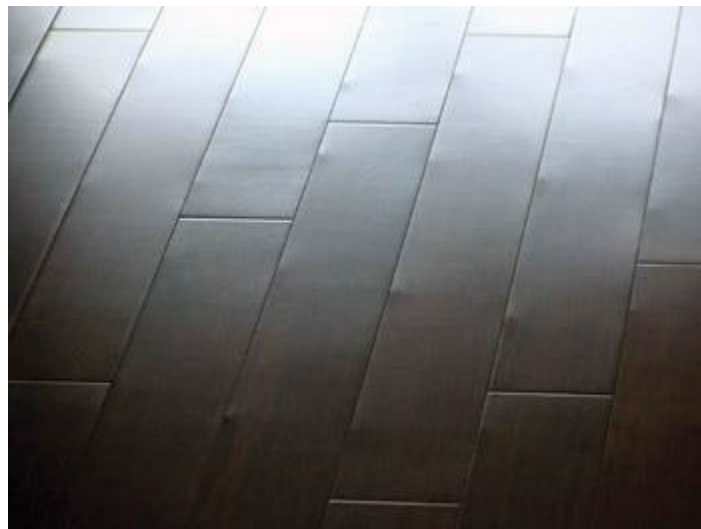
Picture below shows dimpling caused by using improper cleat size
